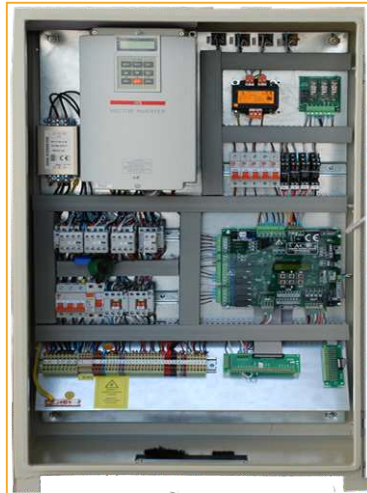
Aybey Elektronik Control Panel
